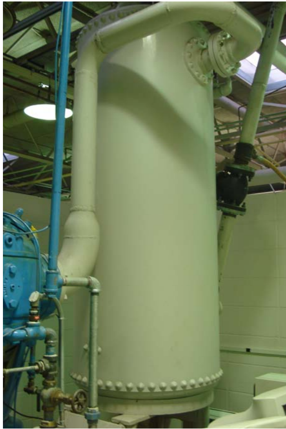
Figure 1: The existing compressed air tank at the Mechanical Engineering building at the University of Arkansas
