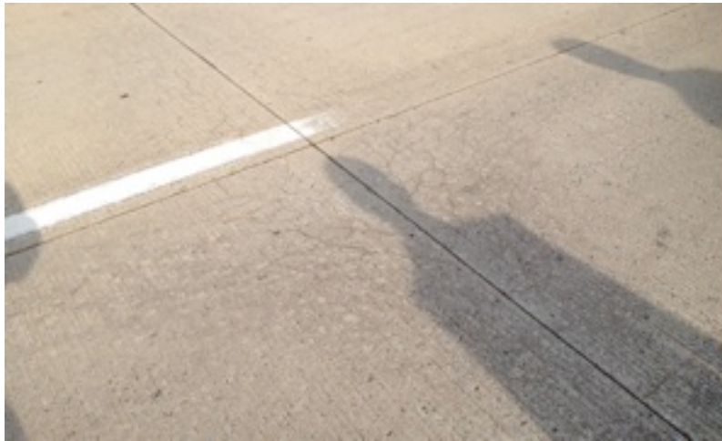
Figure 1. Map cracking in pavement.
