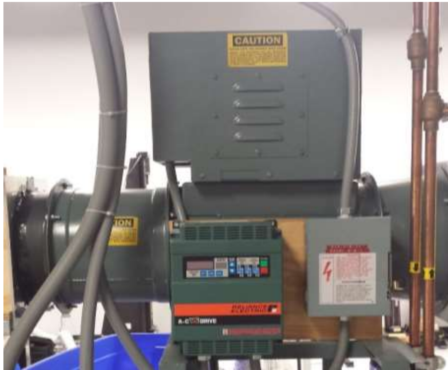
Figure 1 : 2-hp Reliance Electric fan
