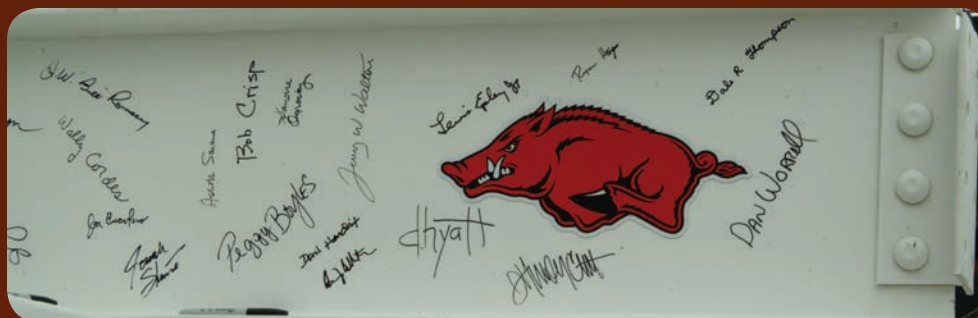
Attendees of topping out ceremonies leave their mark by signing a beam before it is lifted into place, signifying the close of phase one of construction.
