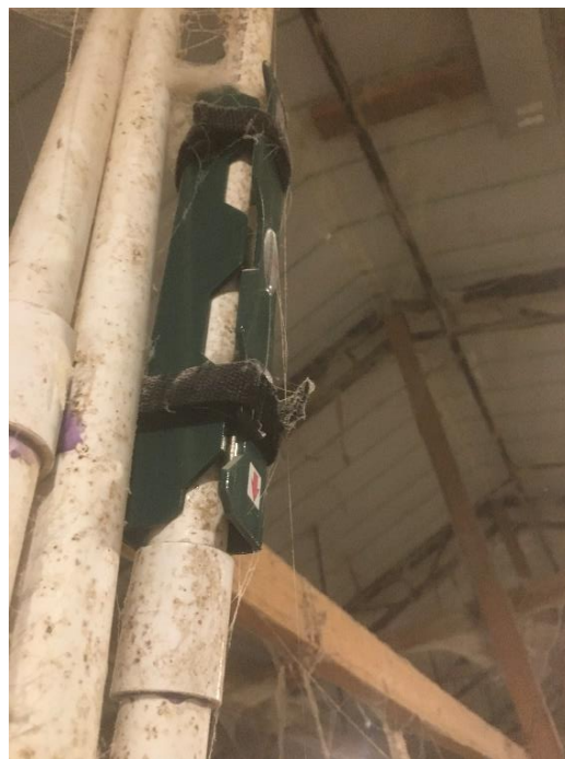
Image 3: Large N52 Neodymium attached to the main pipe
