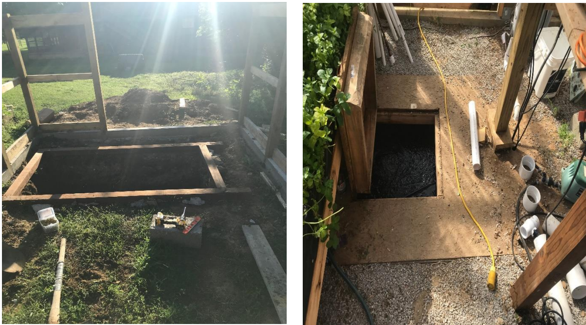
Figure 2. Left to right, initial frame being set on sump tank for fit to complete and covered sump tank with openable hatch. Photo source from Jesse Blanchard.
