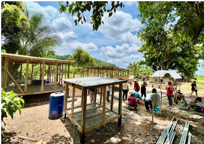
Figure 4. Entire poultry complex except chain link perimeter fence and door on holding pen.
