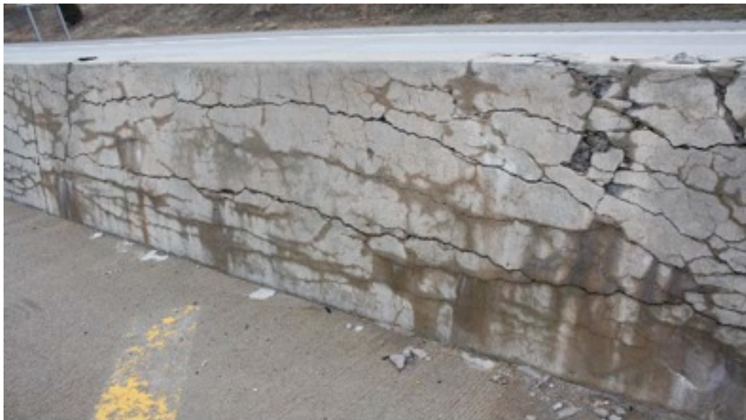
Figure 2. Barrier wall exhibiting ASR deterioration.
