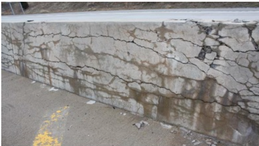
Figure 2. Barrier wall exhibiting ASR deterioration.
