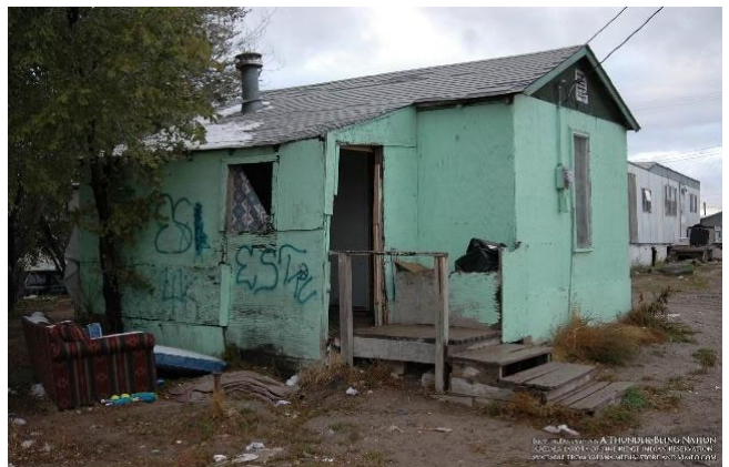
Figure 13. Poor Quality Housing in Pine Ridge
