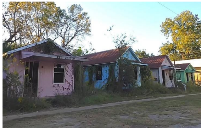
Figure 4. Poor Quality Housing in Dallas County
