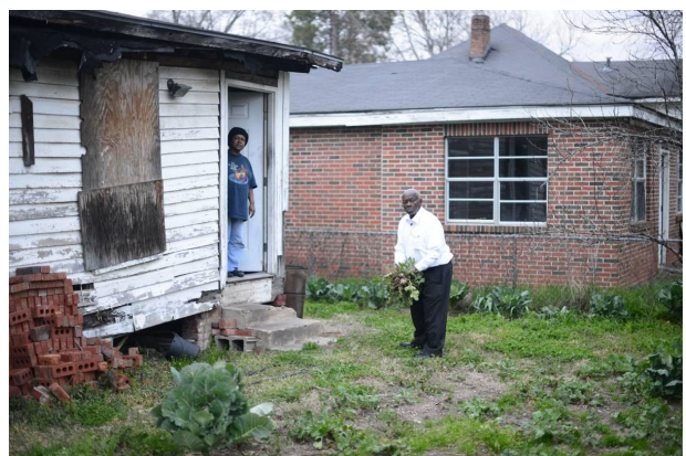
Figure 5. Poor Quality Housing in Dallas County
