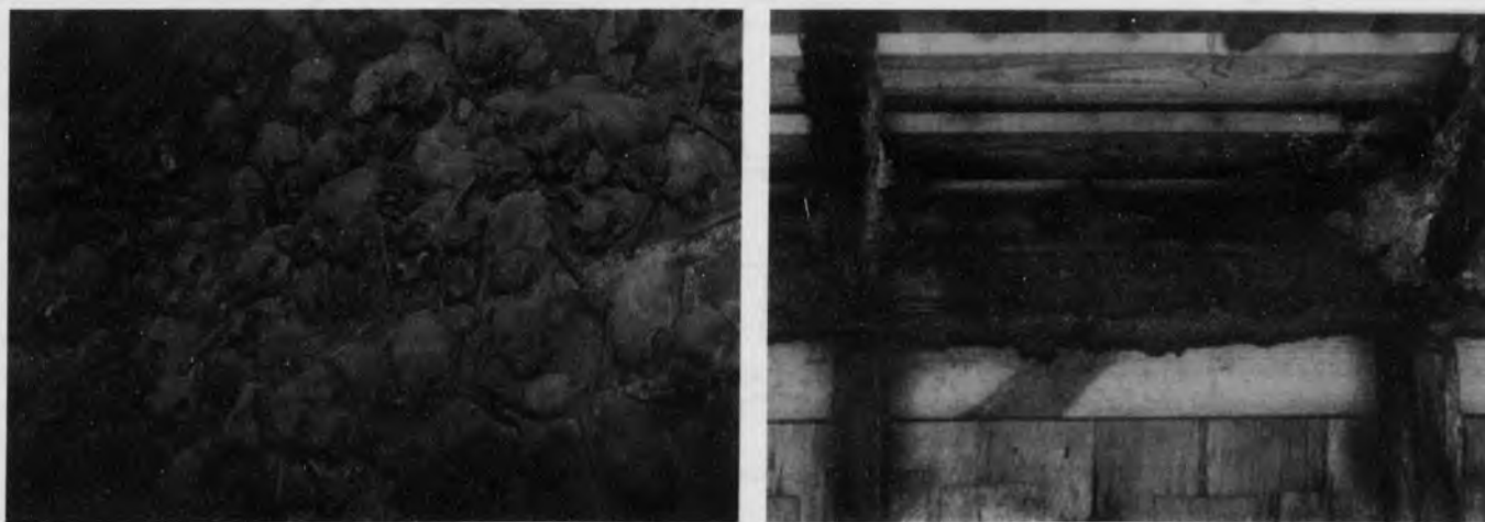
Fig. 3. Free-tailed bat colony roosting in an attic (left) and accumulation of guano (feces) on rafters.
