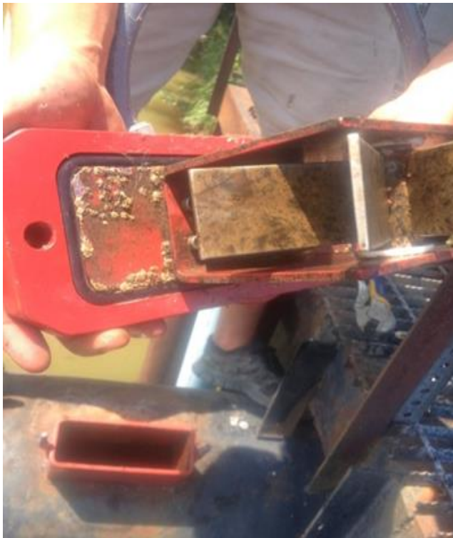
Figure 6. Mineralization and Debris Causing Flowmeter Binding.
