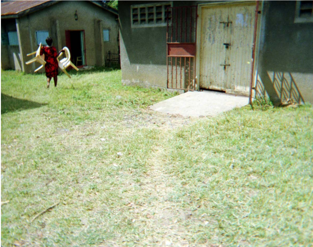
Figure 4.10. The grass path leads into the CBR office. The picture is courtesy of FG1 photovoice session (2015). Note that there is no ramp or specific environmental mobility modification to accommodate the young adults with VI.
