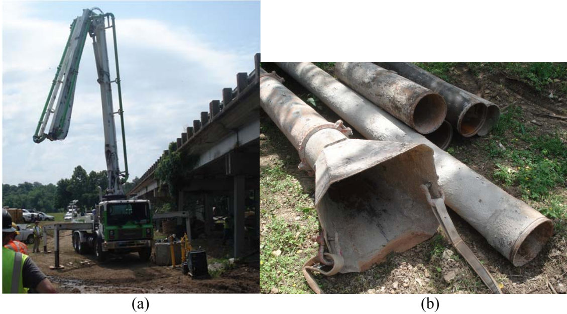
Figure 5.9. Photograph of the concrete placement equipment utilized during construction including the (a) Mantex R-232 concrete pump truck, and (b) tremie pipe.
