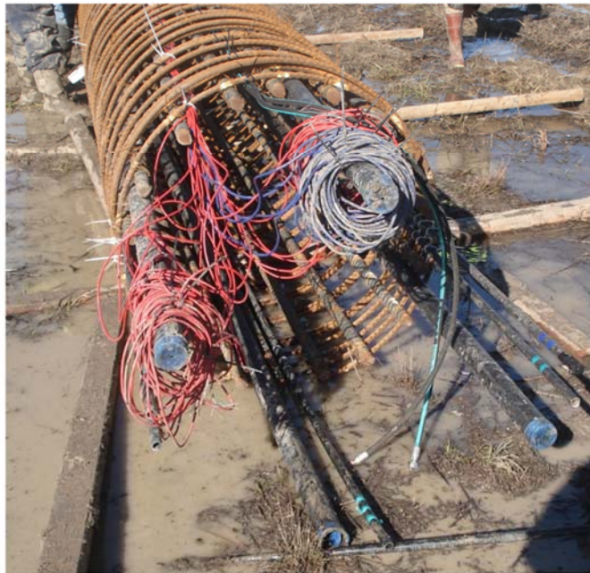
Figure 6.39. Schematic of (a) top-down view of test shaft T-N4, and (b) photograph of instrumented assembly.
