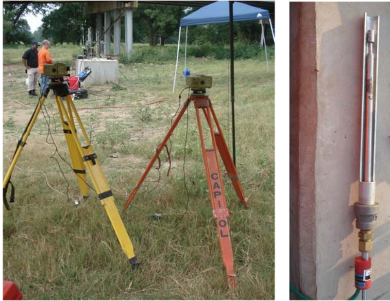
(a) (b) Figure 5.27. Photographs of (a) LVDT displacement instrumentation that was attached to the top of each telltale, and (b) survey levels used to record the shaft head displacement.
