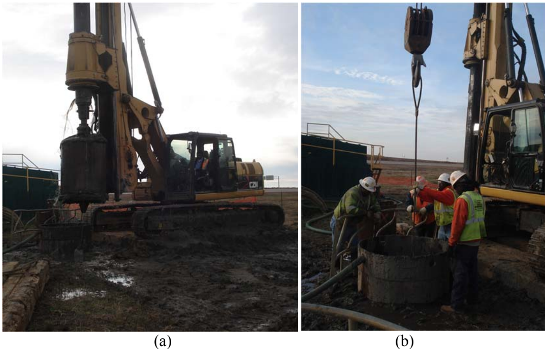
Figure 6.18. Photographs of (a) auger bucket during excavation, and (b) auger bucket retrieval.
