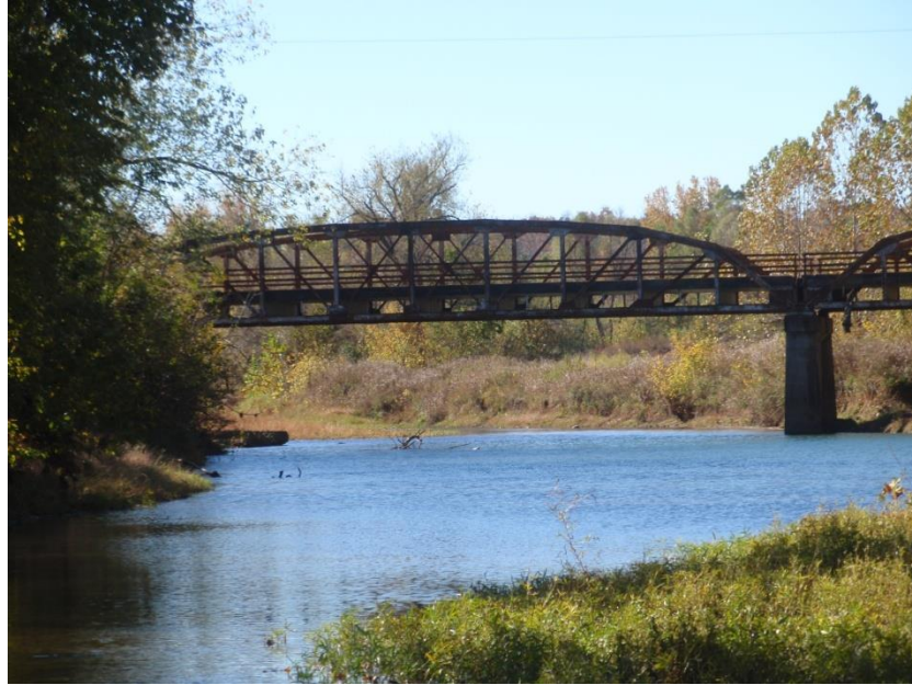
Figure 4.3: Baptist Ford Bridge – Elevation View of Typical Span Photo taken by Jeremy Rawn, Fall 2010 Fayetteville, Arkansas
