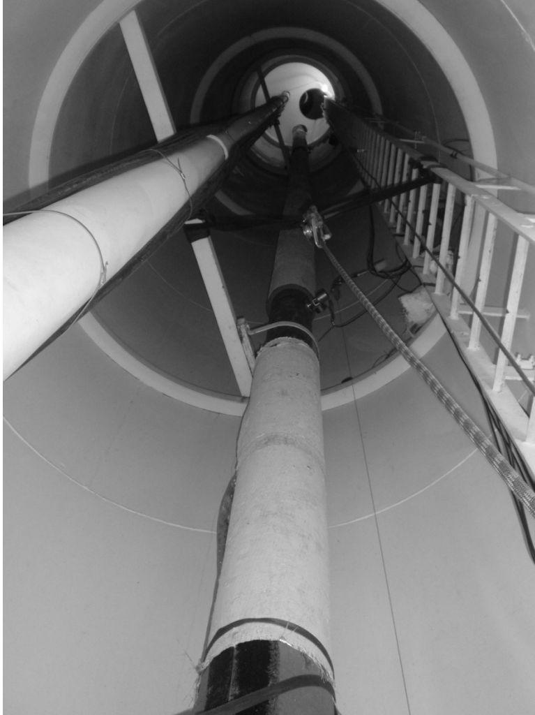
Figure 4.5. Installation of accelerometers on the Elevated Water Tank (Photo by Author)
