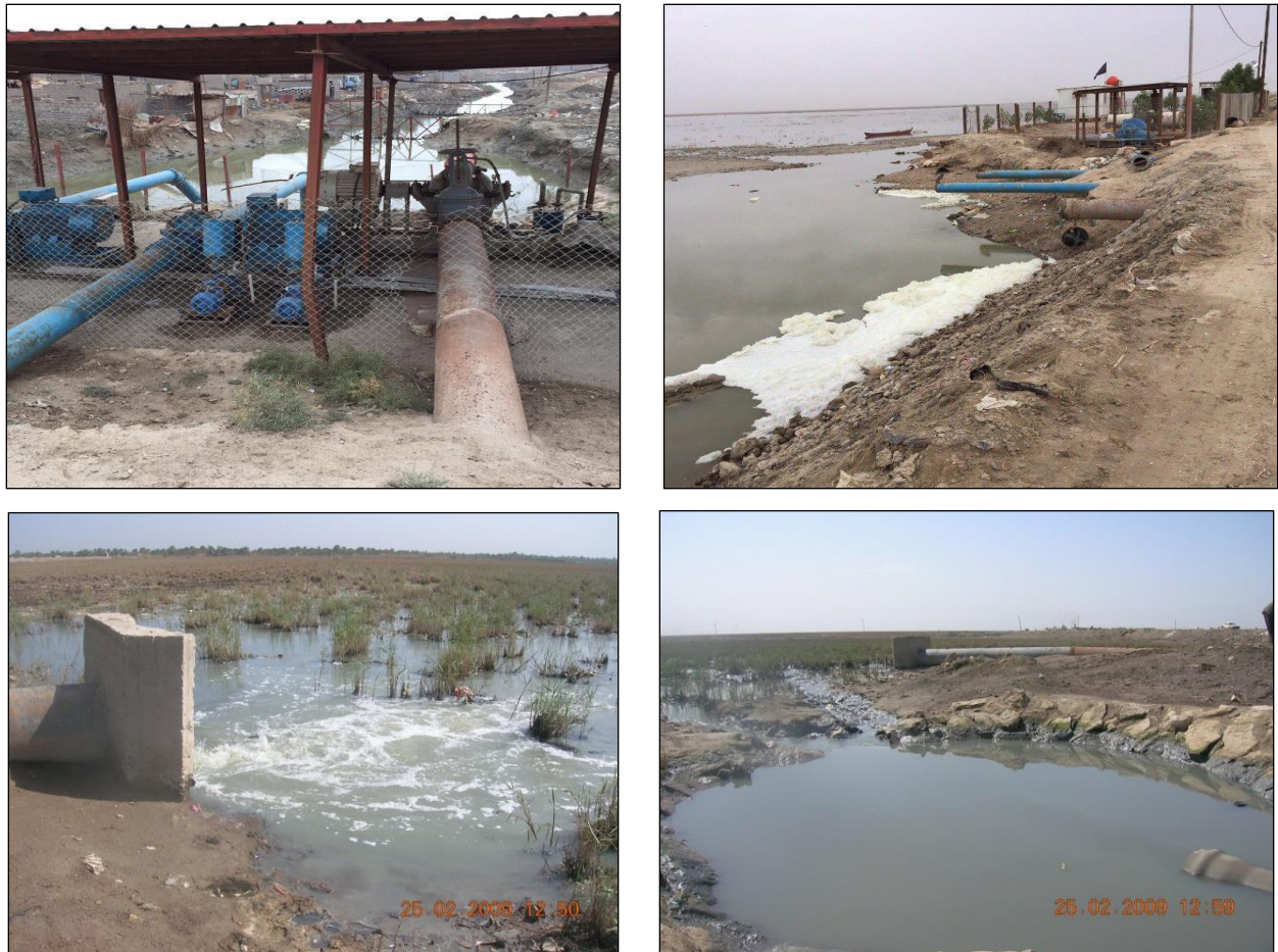
Figure 26. Top- photos of the pipes of the Al-Jaafri pump station, taken by Dr. Jamal Al-Hamdani, 2015. Bottom- photos of the pipes of the Al-Nawashi pump station, taken by Ali Al-Quraishi, 2009.
