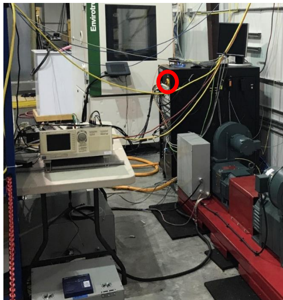
Figure A.9: Power Switch for Data Acquisition System
