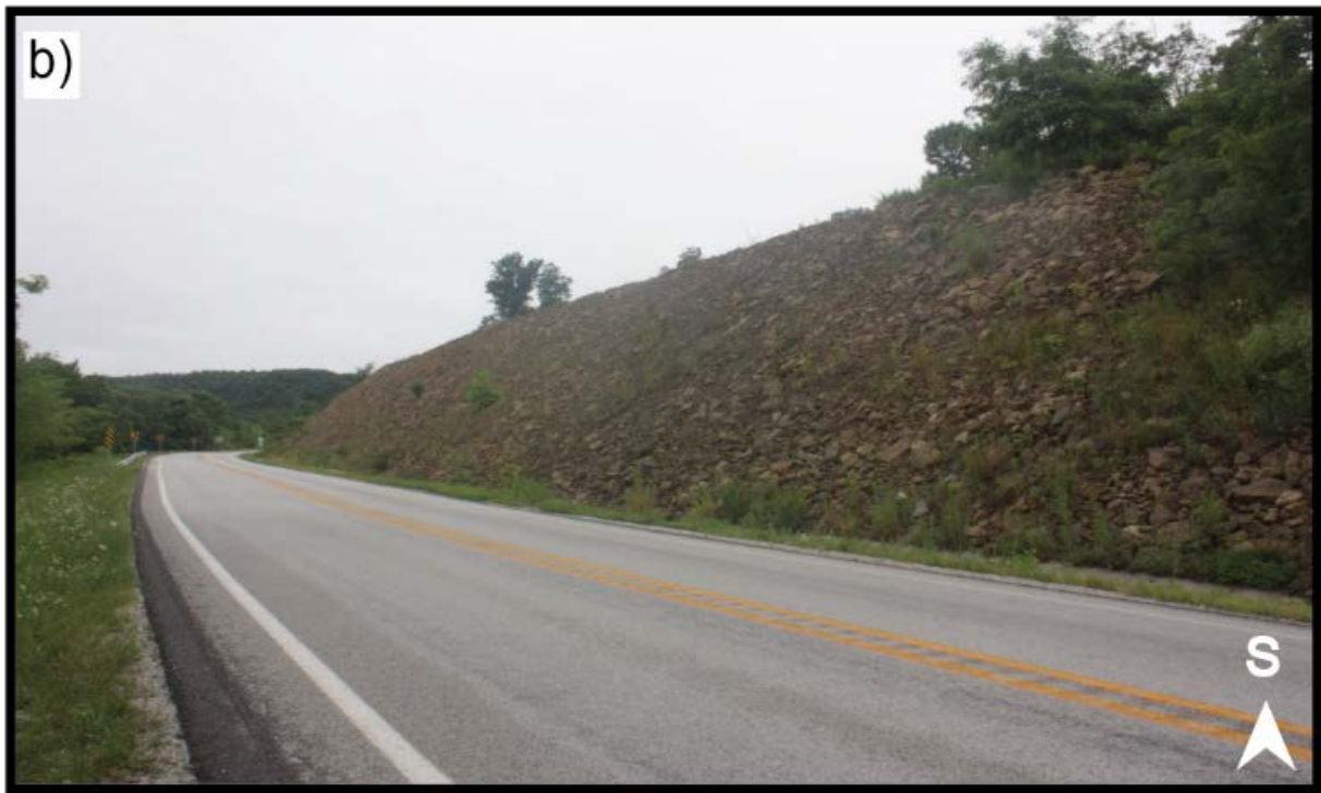
Fig. 5 Riprap with steep angle of repose, part of the most recent mitigation effort to a historically problematic failure zone along Arkansas Highway 7, looking north toward Jasper (a) and looking south uphill (b) with the summit of Round Mountain immediately west
